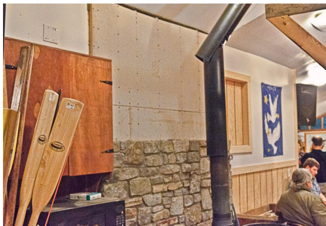
Thank you to John Benjamin and hid band of helpers, Rene Vivo, Saul Roszinsky, and David Eberle for the new stone wall.
